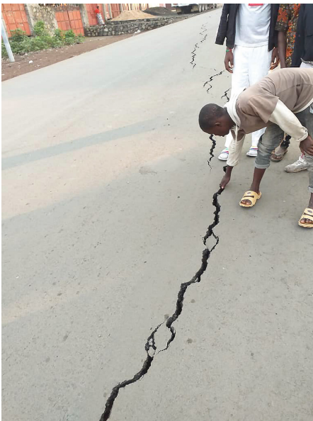
Cracks in roads
