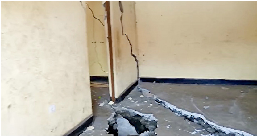
Cracks in buildings
